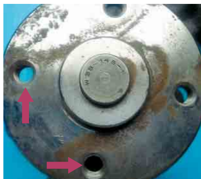
Damage at the stud bolt ends
